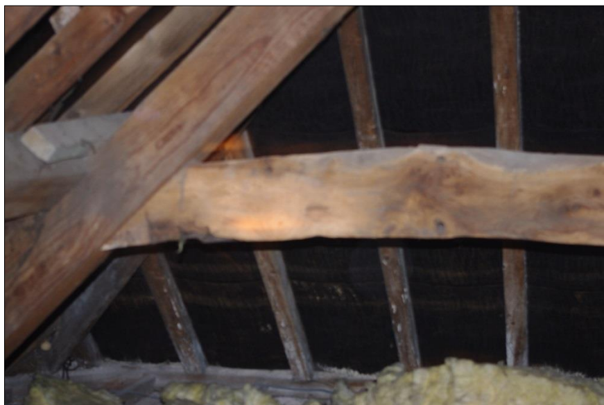
The cross-beam appears to be un-machined. Note contrast with the machined ones.
